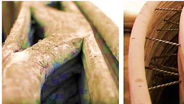
Fig 4. Building a House Using the Apis Cor Robot and its Building Technology.
